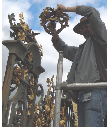
Simon Doyle removes one of the crowns with failing fixings.
